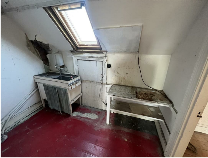
Landing/former kitchenette area with Velux window and access to under eaves storage. Door to
